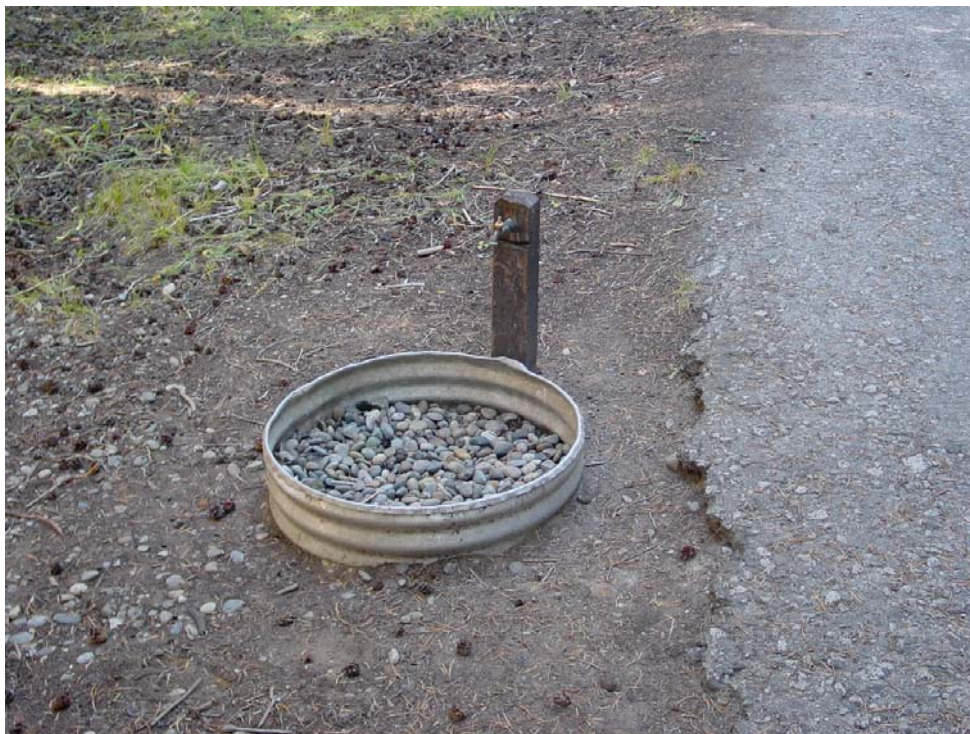
Rancheria Campground, Water Spigot – Non-ADA Compliant Design
