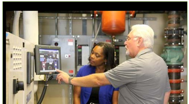
City of Rancho Mirage Facility and Fleet Manager Bill Oppenheim and SCE Account Manager Maya Aubrey review the monitoring system for the smart chiller at the City Library. The city received a $15,000 SCE incentive toward the purchase of the chiller, which reduces energy use by approximately 20% to 30% compared to the older unit.
