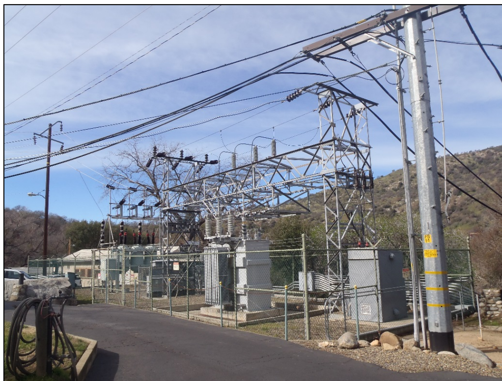
Figure 3.12-1f. Kaweah No. 1 Switchyard.
