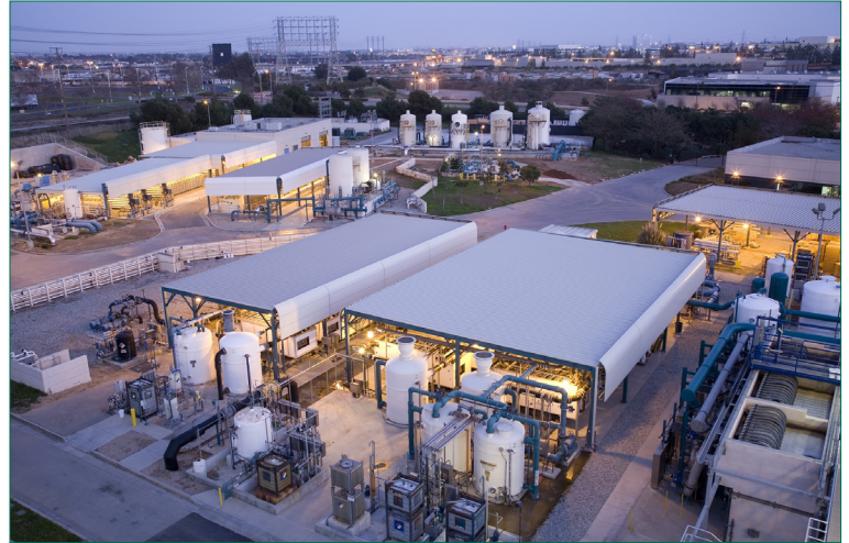
System improvements at West Basin Municipal Water District's Edward C. Little Water Recycling Facility are improving efficiencies and enabling reduction of more than 1 megawatt of load for demand response participation.
