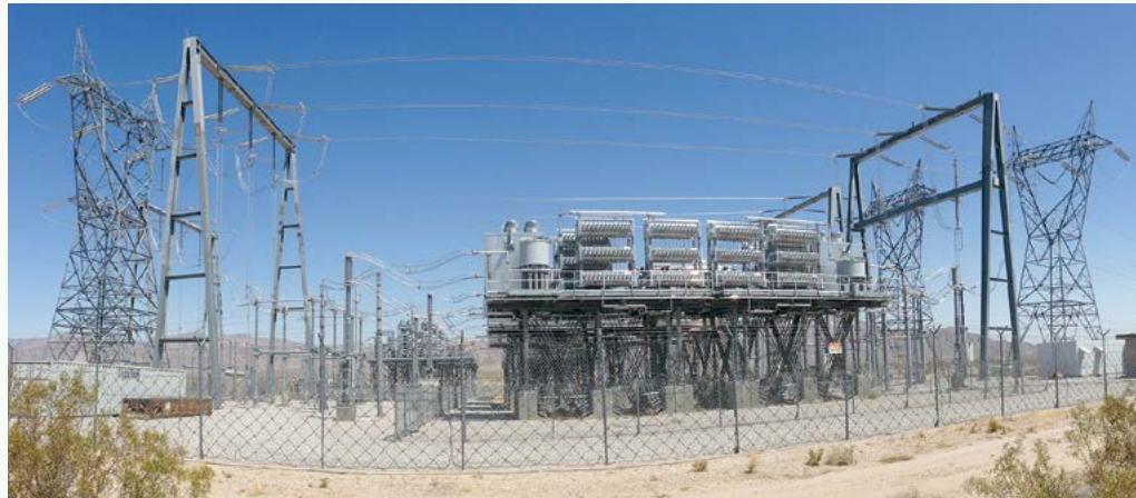
A capacitor bank (middle of photo) helps electricity to pass efficiently across long distances.
