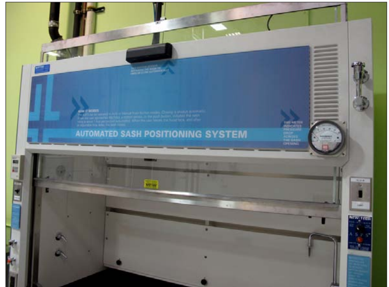
An automated sash positioning control system helps conserve energy by closing the sash to reduce the exhaust and makeup air flowing through the fume hood, when the fume hood is not in use.
