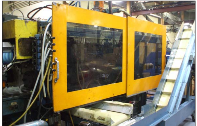
This King Plastics injection molding machine, along with two others, features a new induction heater that uses about 30% less energy than the previously installed resistance heater. The company received an incentive for the induction heaters through SCE's Standard Performance Contract Program.
