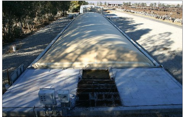
Meadowbrook Dairy uses a plug-flow digester (with the covered digester tank shown here) to generate electricity from cow manure. The digester connects to the electrical system through SCE's Net Metering Program.
