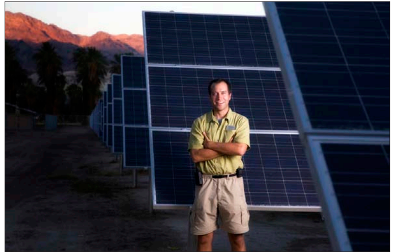
Joel Southall, director of environmental health and safety in Death Valley National Park for Xanterra Parks & Resorts, standing in front of the site's 1-megawatt solar energy generating system, said, "We focus on balancing economic viability with ecological responsibility. Our success lies in surpassing guest expectations while achieving energy savings."
