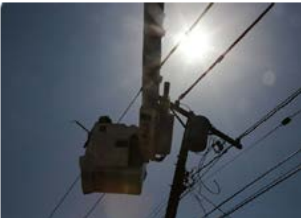
An SCE crew makes repairs during a heat wave. Credit: Jean Anderson
