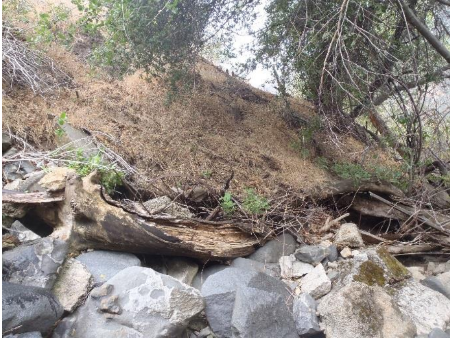
Figure AQ 5-7c. Representative section of the natural drainage channel that receives flow from the Kaweah No. 3 Forebay showing boulders along the side slopes of the drainage.
