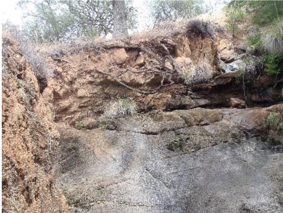
Figure AQ 5-6c. Recent erosion on the side slope of the natural drainage channel which receives flow from the Kaweah No. 2 Forebay.
